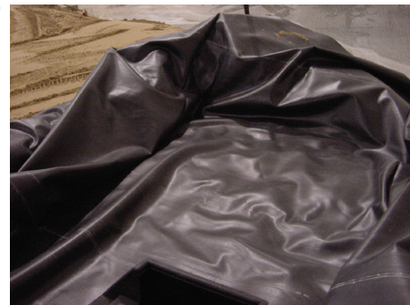
The liner covers the stream bed and goes through the area where the spillway will sit.
